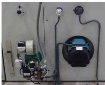
DUAL-HEAT system combines gas and thermal oil.
