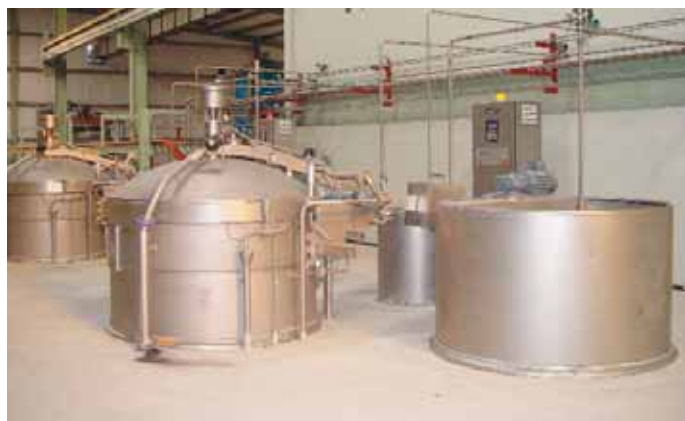
Fong's ALLWIN Package Dyeing Machines installed at Interloop's Dye-house.
