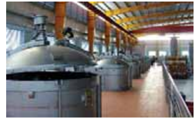
Figure 3: Fong's ALLWIN High Temperature Package Dyeing Machines installed at Knit Concern's well-appointed plant.
